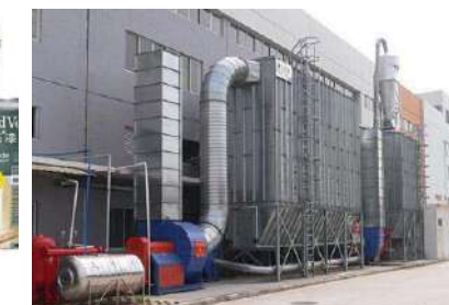
配套除尘系统 Factory dust removing system
